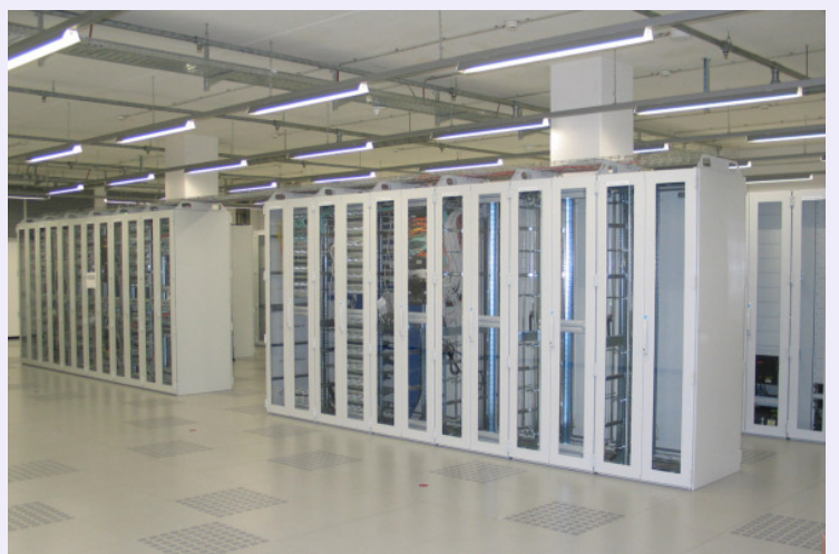
HUK-COBURG installed a total of 75 new, closed IT racks from Rittal in the new "RIO" data centre
