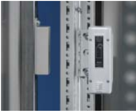
The wireless access sensor reports any unauthorised access.
